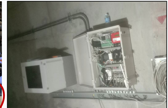
▪ DAQ not properly sealed
